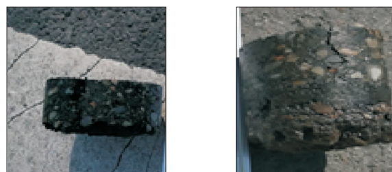
(a) S223 K30+113纵缝处芯样 (b) S223 K31+340横缝处芯样
